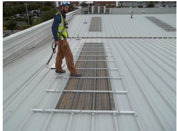
Rooflight Cover (and roof with fall prevention cable system)
